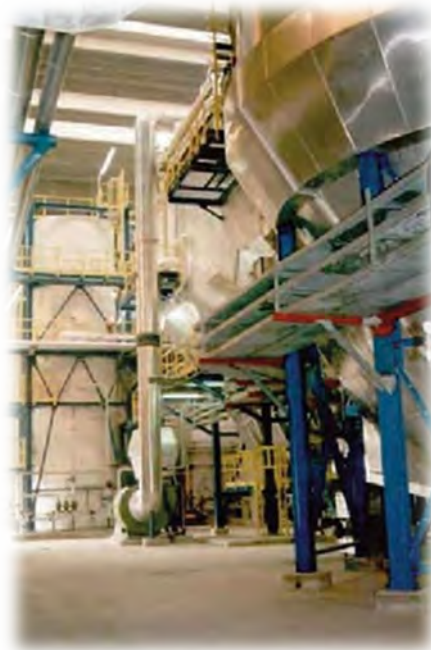
Busto Arsizio waste to energy plant
