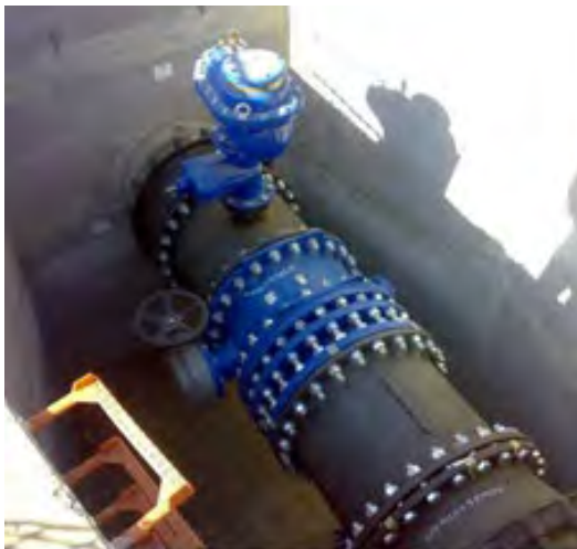
Detail of the main pipe
