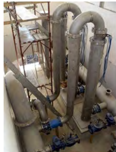
Detail of a pumping station
