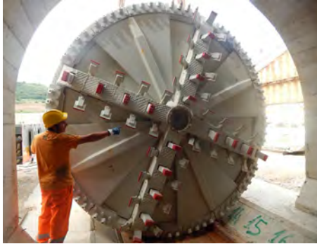
Detail of the TBM
