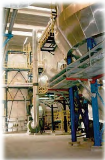
Busto Arsizio waste to energy plant
